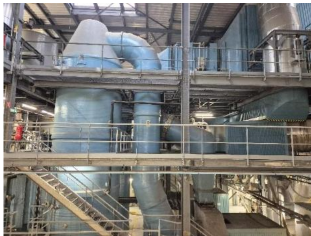
Figure 14 – Colonne de lavage
